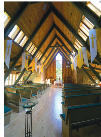
The St. Benedict Chapel got a new roof, windows, insulation and other improvements in 2005. (Kristen Hannum/Catholic Sentinel)
